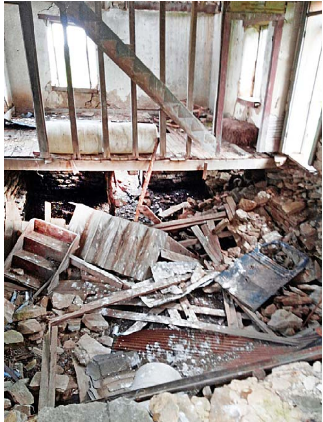
Looking through the parlor window, the parlor floor is gone. The front entry is to the right and you can see the right side of the staircase and pieces of the stair in the basement. The floor of the family room is on the far side.
