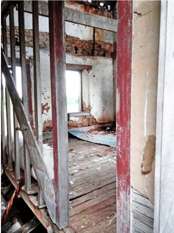
Looking in the front door to the right is the area you described as the family room. You can still see some of the flooring there, but I don't think I would want to try walking on it!
